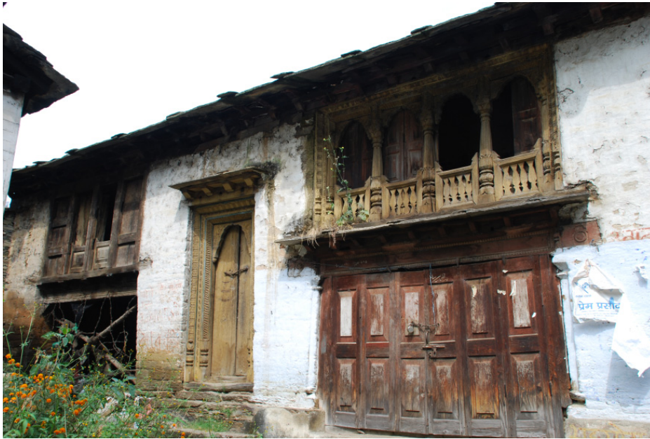
Figure 2: Photograph depicts physical, chemical, and biological deterioration of vernacular architecture materials.
