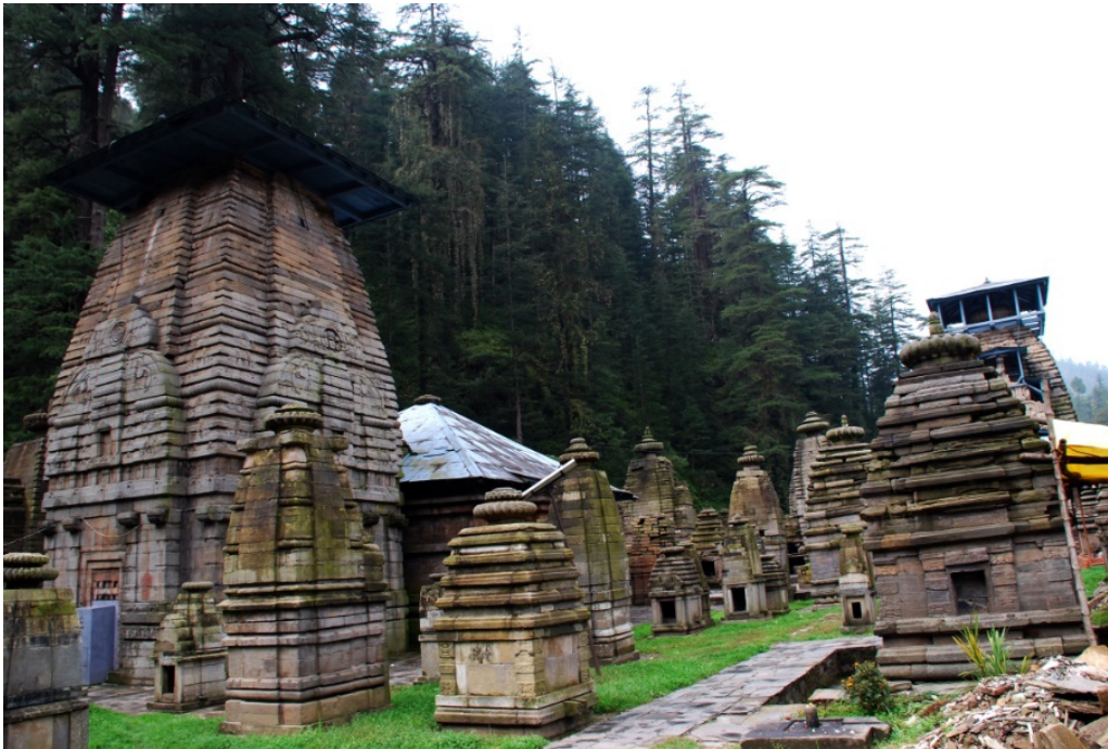
Figure 7: The picture shows various problems with the stone including cracking, fading, algae, moss, fungus, lichen, vegetation, dirt, biological deterioration, breakage, calcareous deposition, deterioration caused by bird excreta, human vandalism, soot, and soluble salts.
