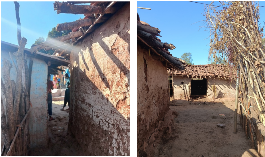
Figure 3: The image displays wall deterioration caused by water capillary action, dust and dirt accumulation, stains, vegetation, bird excreta, insects, fungus, mud wall cracking and chipping, human negligence and vandalism, as well as fading due to atmospheric gases and pollution.
