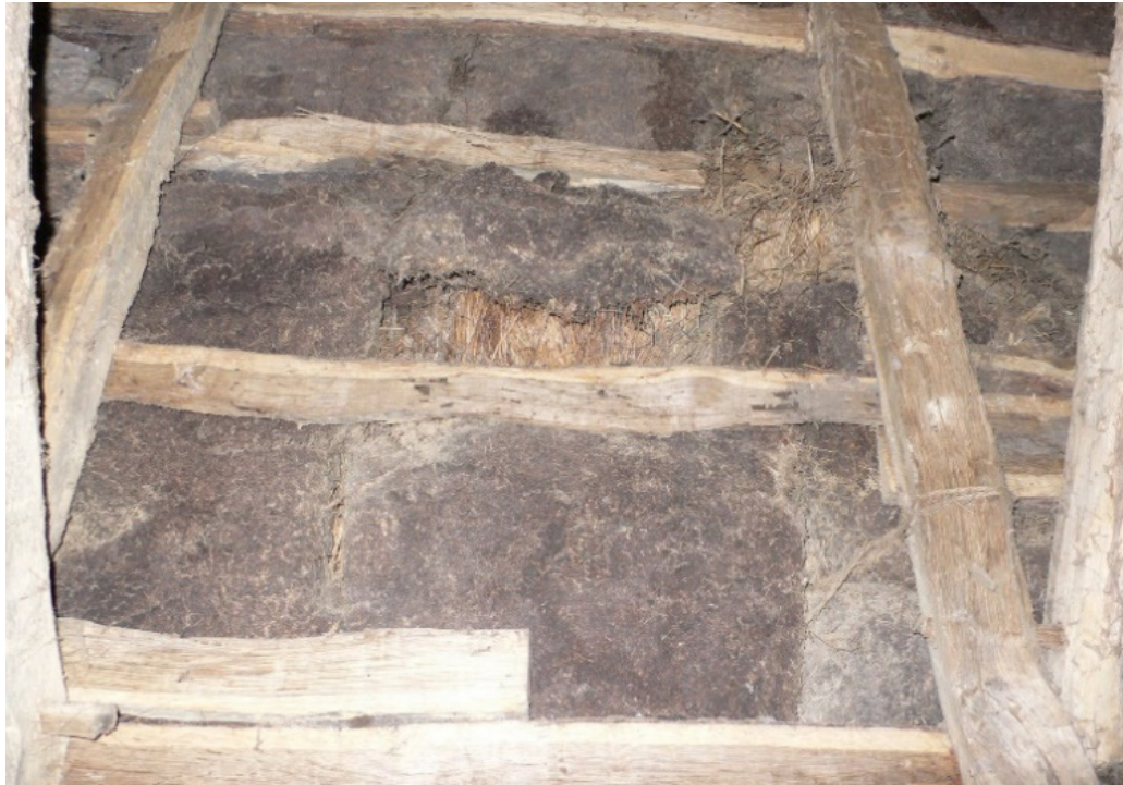
Figure 4: Underside of roof, near Killorglin, County Kerry, showing scraw (turf underthatch), with some straw showing through (in the middle of the image)
